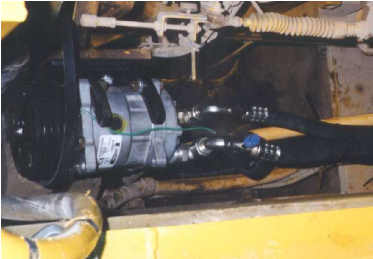
Compressor and mount in place on engine. View from top of engine compartment.
