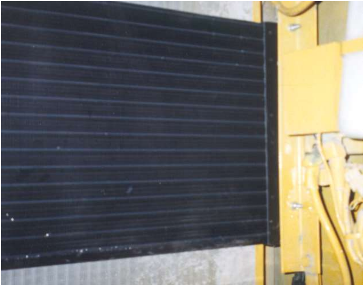
Right side of condenser with bolts in place through flange.
