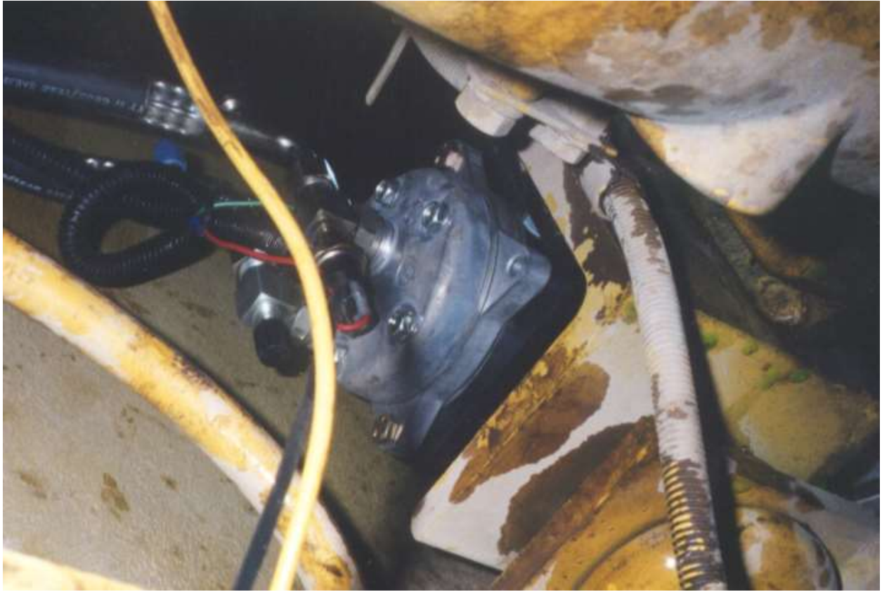
Compressor in place. View from underneath.
