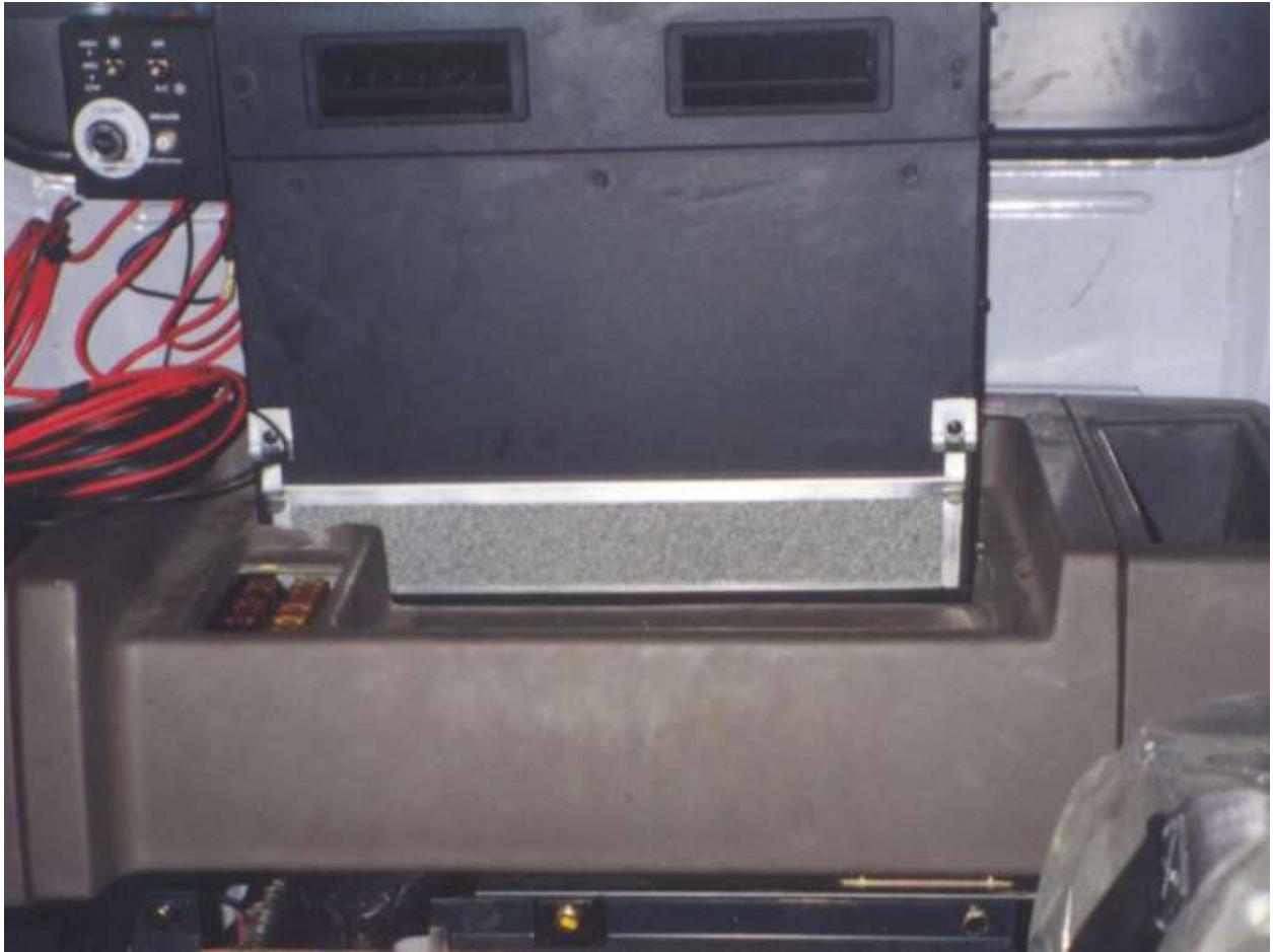
Evaporator in place on back wall of cab. Note that it extends above the lower window line.
